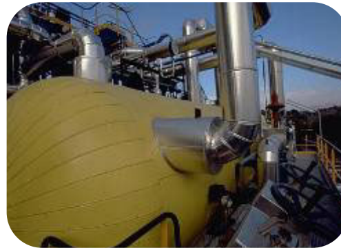
PA 11 monomer production units in Marseille (France)
